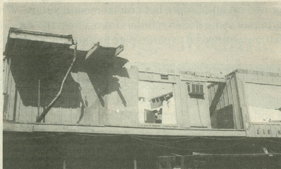
The roof was ripped from the Westmoreland Square Apartments, 219 Marshall, and several units were gutted when a tornado struck suddenly in Montrose on November 16. (Photo by Amber Ratisseau)
